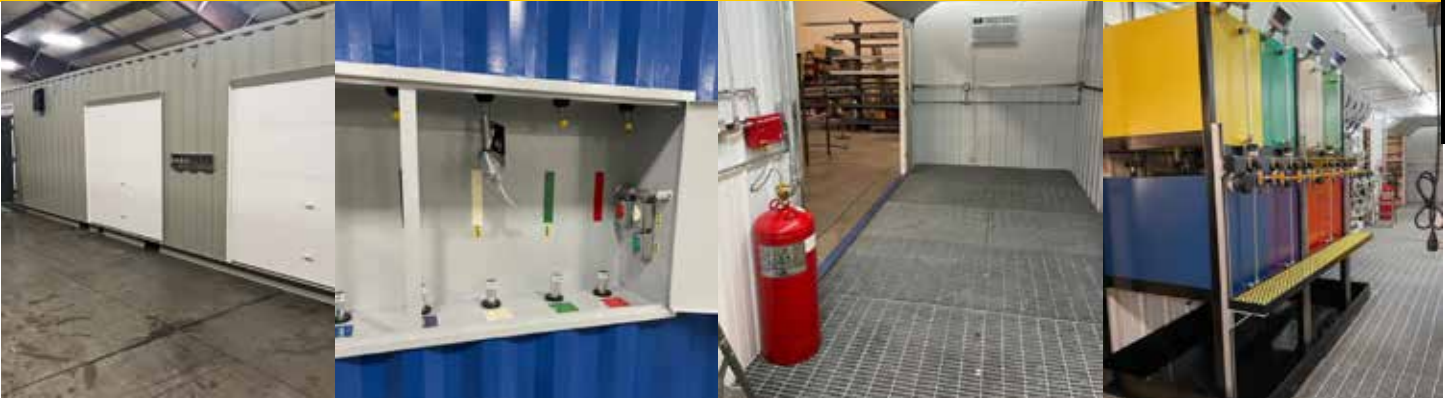
40 FT x 8 FT Room with 2 Roll-up Garage Doors
